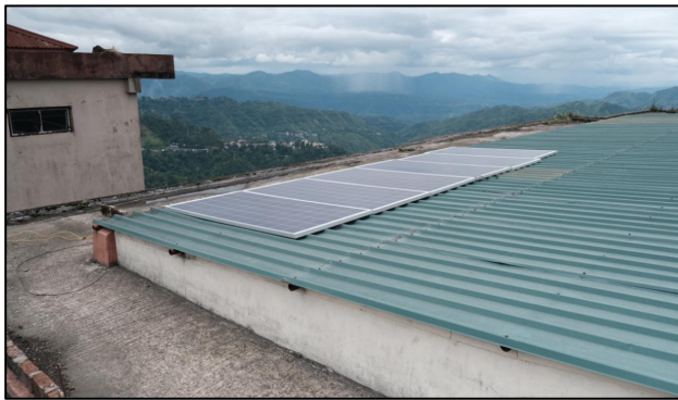
Rooftop Solar Panel
