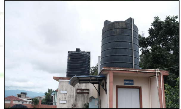
Rooftop Water Storage Tank
