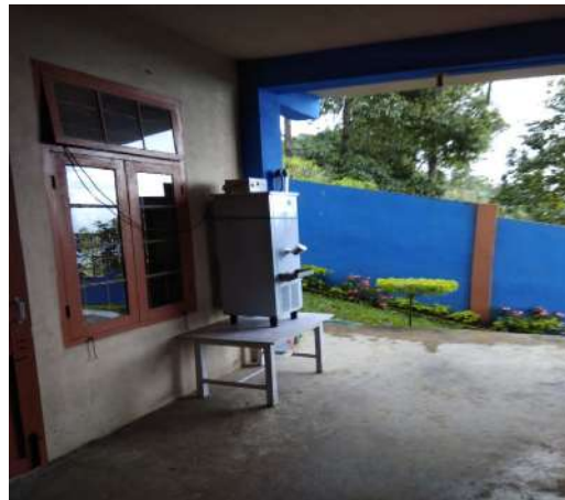
Photo20: Water Cooler at Women Hostel
